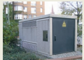
Medium-voltage local network station
