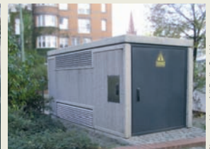
Medium-voltage local network station
